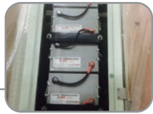
Battery Maintenance Free Battery
